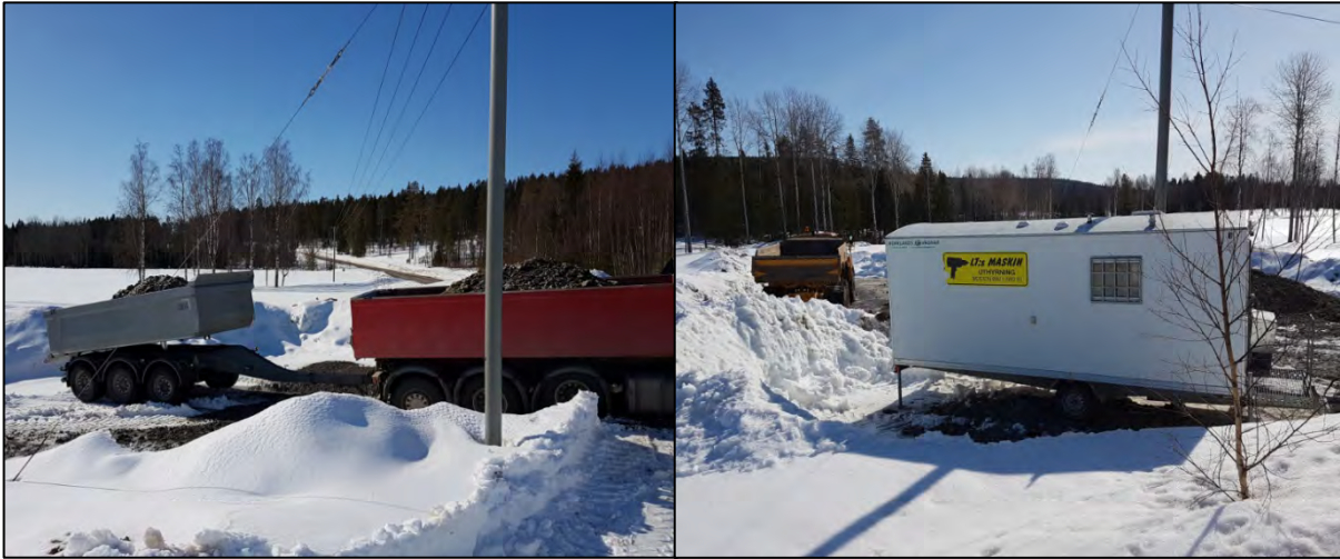
Figure 4.22. Transporting material for reloading onto a dumper truck (picture on the right).
