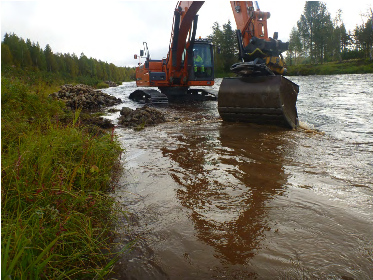
Figure 2. Stone material ready to be used for making a rocky salmon-fry area at Mötyskoski.
