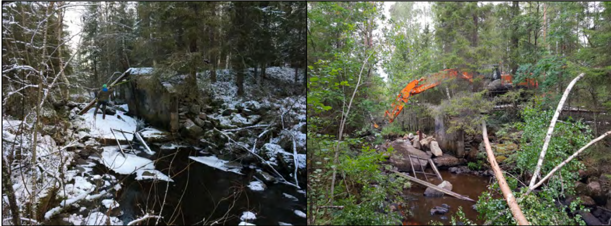
Figure 4.6. Baronseldammen dam in the Rosån river prior to work being undertaken. Concrete and metal structures were removed from the watercourse and from both banks.
