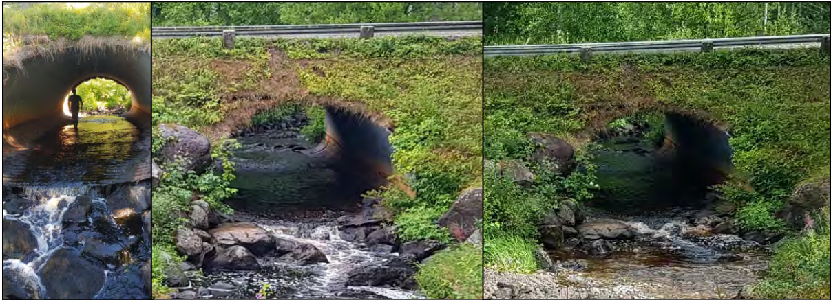
Figure 4.14. Rosfors, road culvert in the Rosån river. The two pictures on the left are before the work was carried out and the picture on the right is after the work was undertaken.
