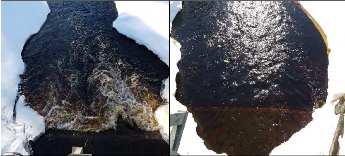
Figure 4.24. The picture on the left is before work was carried out and on the right after work was carried out at Selets Bruk, Alån river. After the work was carried out the water level below the dam was raised, creating a free migration route for fish (picture on the right).
