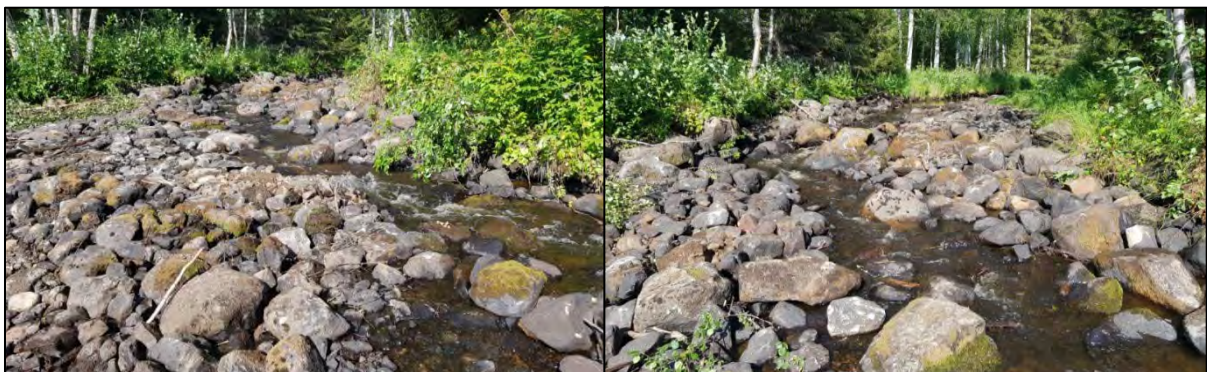
Figure 4.10. The picture on the left shows the middle section of the weir following the work and the picture on the right shows the upper section of the work. On the day that work was carried out the water flow was extremely low, about 5 litres/s.
