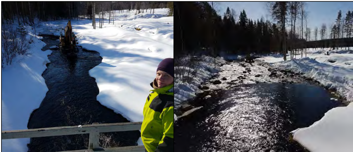
Figure 4.23. The picture on the left shows the transport of material by an excavator into the main channel of the Alån river, and the picture on the right shows the arrangement of rock in the works area.
