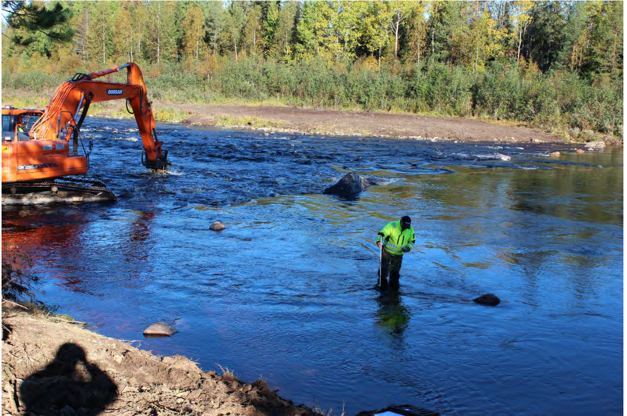
Figure 1. Water current speed and riverbed depth are measured in connection with the restoration work.
