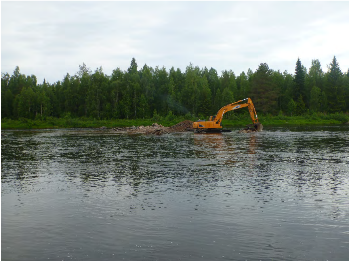
Figure 5. Sifting of stone material in connection with the demolition of the small jetty at Maitokalliovirta.
