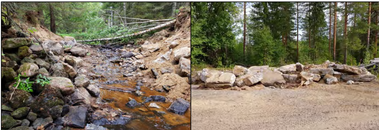
Figure 4.7. Baronseldammen dam, Rosån river after work to create a modified channel for migrating fish. The concrete material on the right was transported to landfill. There was an extremely low water discharge (about 3 litres per second) when the work was carried out.
