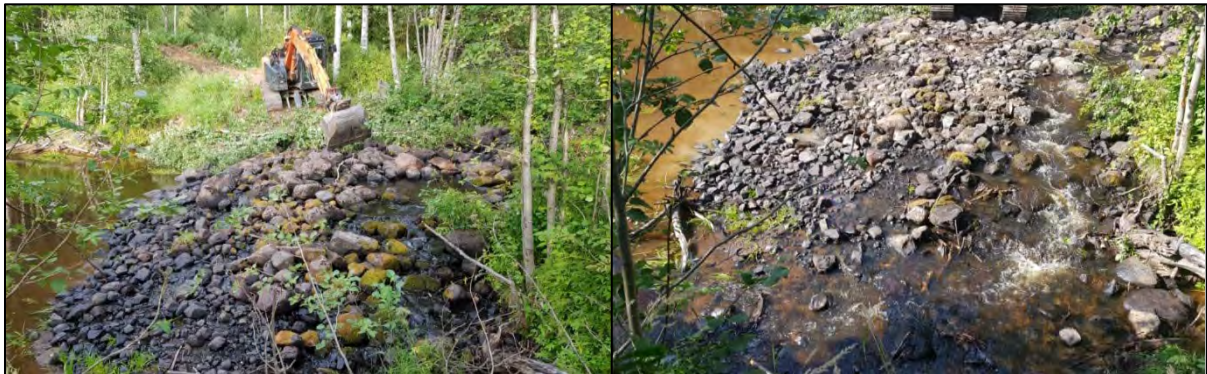
Figure 4.9. The picture on the left shows the weir before work was carried out, and the picture on the right shows the concentrated channel at the bottom of the rock weir. On the day that work was carried out the water flow was about 5 litres/s.
