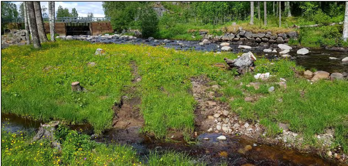
Figure 4.25. Transport route for the excavator and dumper truck at Selets Bruk showing little rutting after the work carried out in April 2018.
