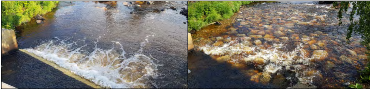
Figure 4.18. The weir at Ale Kvarn in the Alån river before work was carried on the left, and after work was carried out on the right. The water level was very low when the work was carried out.
