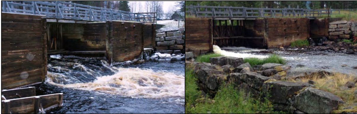
Figure 4.20. The dam construction at Selets Bruk, Alån river. The picture on the left shows the gates open and the picture on the right shows them closed.
